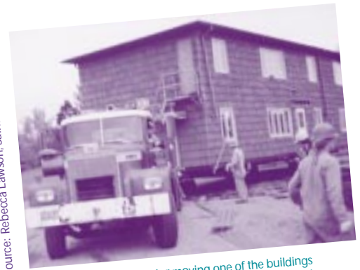
Contractor moving one of the buildings for the Bagley Downs apartment complex
